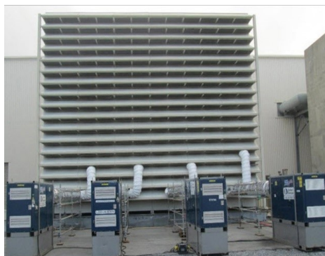
Temporary heaters and ducting Source: ReliabilityFirst Corp.
